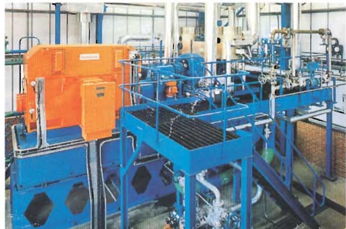
PM40 coupling on a Peter Brotherhood steam turbine generator.
