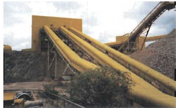
Conveyor drives. Couplings fitted on belt conveyor drives.
